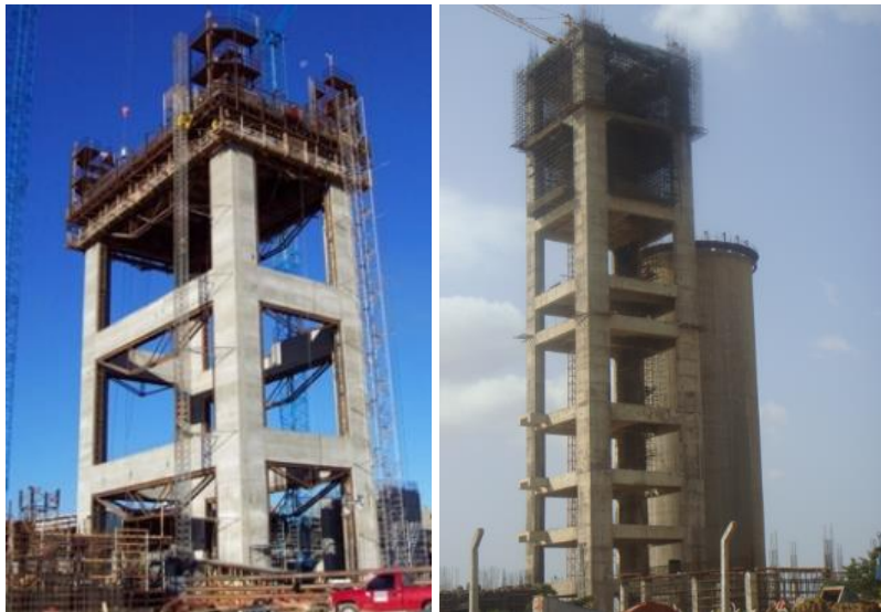
Fig. 4: –Value Engineering – Slip-form (L) vs jump form (R) – Construction time savings 5-7 months
