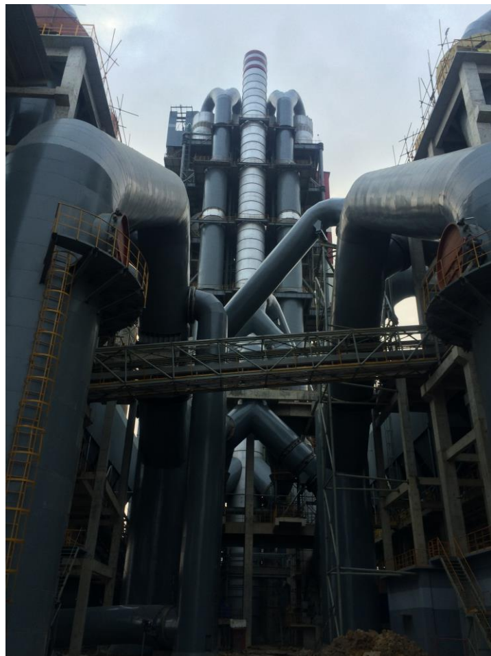
Fig.2: Typical view on a down comer duct spray installed between preheater and raw mill section,
