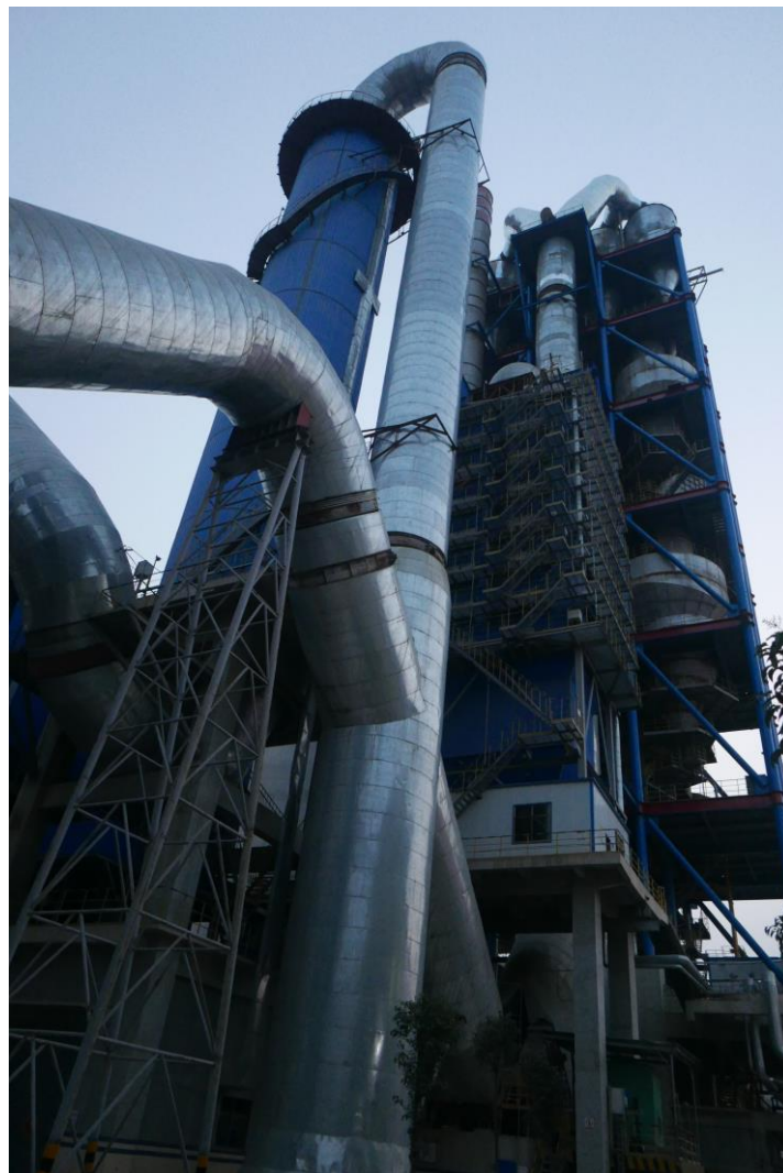
Fig.1: Typical view of a GCT system installed between preheater and raw mill section.
